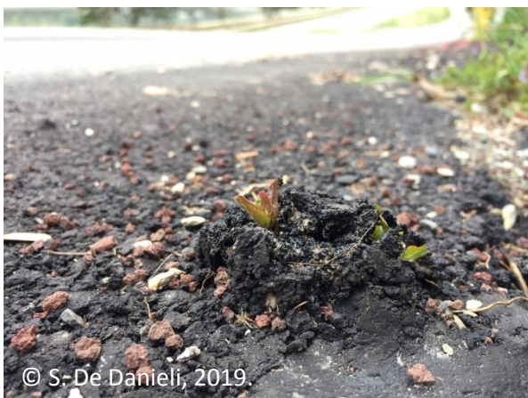
Figure 10. Regenerating ramets of knotweed growing through a freshly resurfaced road in the French Alps near Grenoble. As no knotweeds grew there before the surfacing works, fragments of the plant must have been brought by the heavy equipment used for the works.
