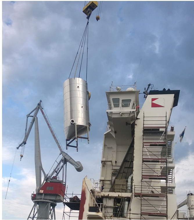
(a) Installation of an exhaust gas treatment plant: a scrubber, from [25]
