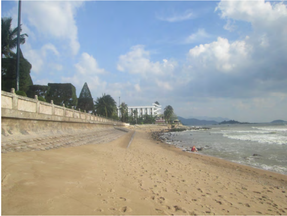
Figure 2.14: A part of the vertical and sloping seawall along the stretch between Nha Trang View restaurant and the structure Hoa Bien.
