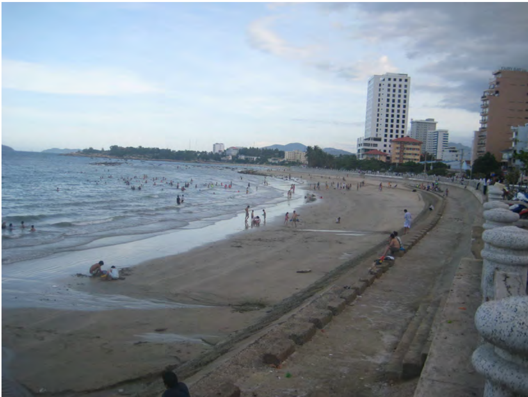
Figure 2.5: The beach of Cai river mouth has suffered from severe erosion and today the beach is absent and only the seawall is visible. Photo taken at 16h51 24/05/2013.
