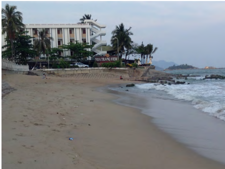
Figure 2.12: The seawall and the groins at the beach south of Nha Trang View restaurant. Photo taken at 11h14 12/03/2015.
