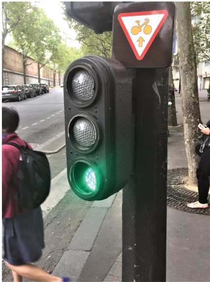
(A) Faulty Traffic Light
