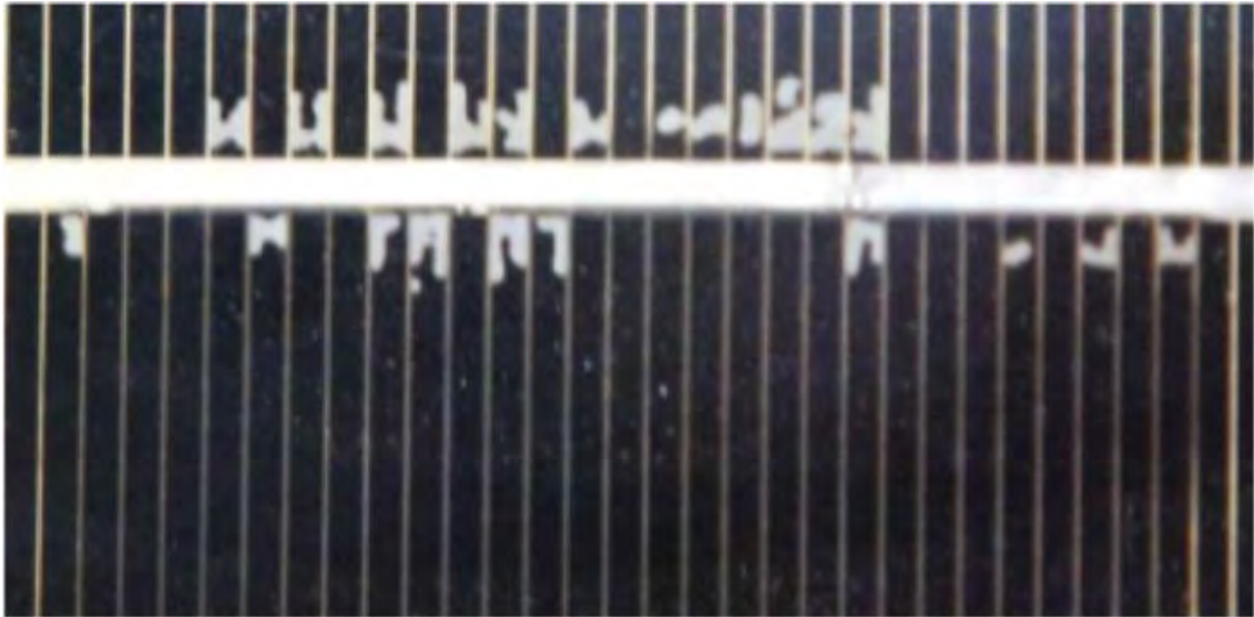
Fig. 45 Delamination at the cell-EVA interface in the proximity of the interconnection ribbons.
