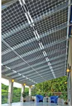
Patio Awning: Solar Living Design Lakewood, CO
