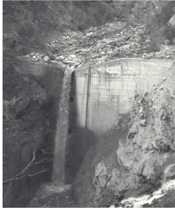
Figure 1.4 – The 34-m-high ‘Fèvre’ check dam in the Bonrieu branch of the Saint Martin torrent (73 - FRA.); 4-m-thick at the crest, 7.6-m-thick at the toe, construction: 1939-1942, just upstream of the huge lateral Bon Rieu landslide (Messines du Sourbier, 1939a). The downstream gorge is currently filled by the landslide movement, stabilizing it. The dam is still in good condition, almost completely buried by the landslide, and it fulfills its function perfectly: decrease the energy and erosive power of debris flows upstream of a reach whose incision has catastrophic consequences (photo Apr. 1955 by L. Ancherri courtesy of RTM73).
