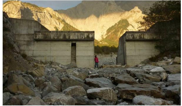
Figure 2.10 – Downstream view of the slit dam on the Ebron torrent (Tréminis (38), FRA), the initially triple small slit dam built in 1990 (see one obstructed slit on the left) has been cut ca. 1998 to become a large slit dam. This operation having deteriorated the structure strength, a big rip-rap layer fixed with concrete has been added on the dam upstream side to increase the structural resistance to debris flow impact. (image by Guillaume Piton)
