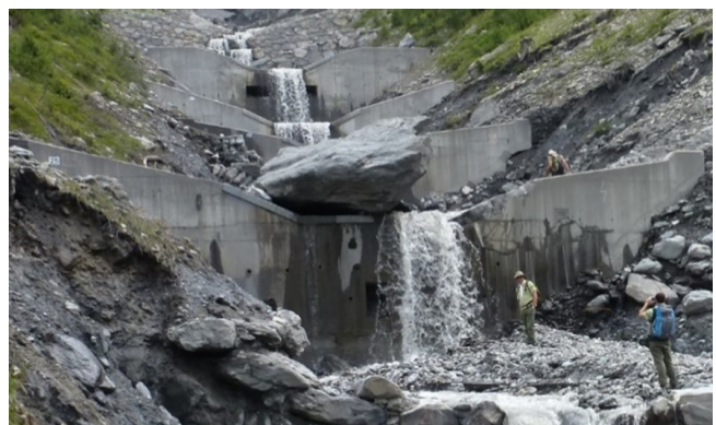
Figure 1.10 – Huge boulder stopped on the check dam series of the St. Antoine torrent upper basin (73 – FRA.) – 2014 (photo courtesy of S. Carladous)
