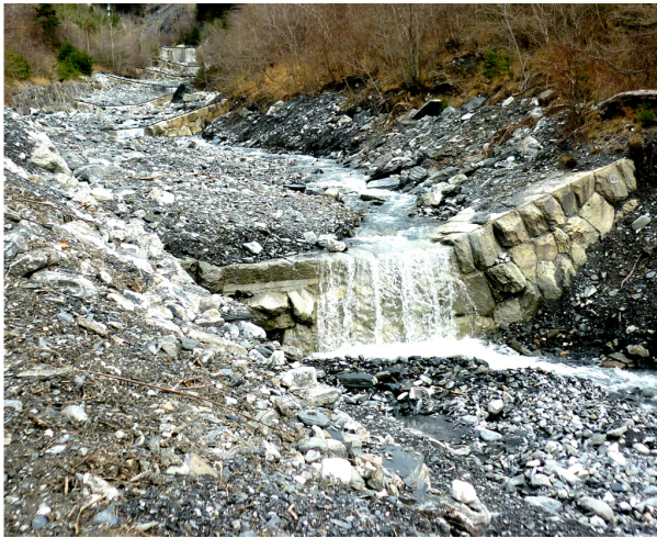
Figure 5.1 – Check dam series in the Saint Julien Torrent (73) Fr – 2015, grade control structure built above the bed level (photo courtesy of S. MEJEAN)
