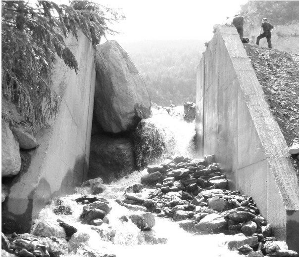
Figure 2.5 – Downstream view of the St Antoine sediment trap after the 31 July 2014 debris flows: mechanical blockage of the 5-m-wide, 8-m-high slit dam by three boulders 3-4 m in diameter (image by Guillaume Piton)
