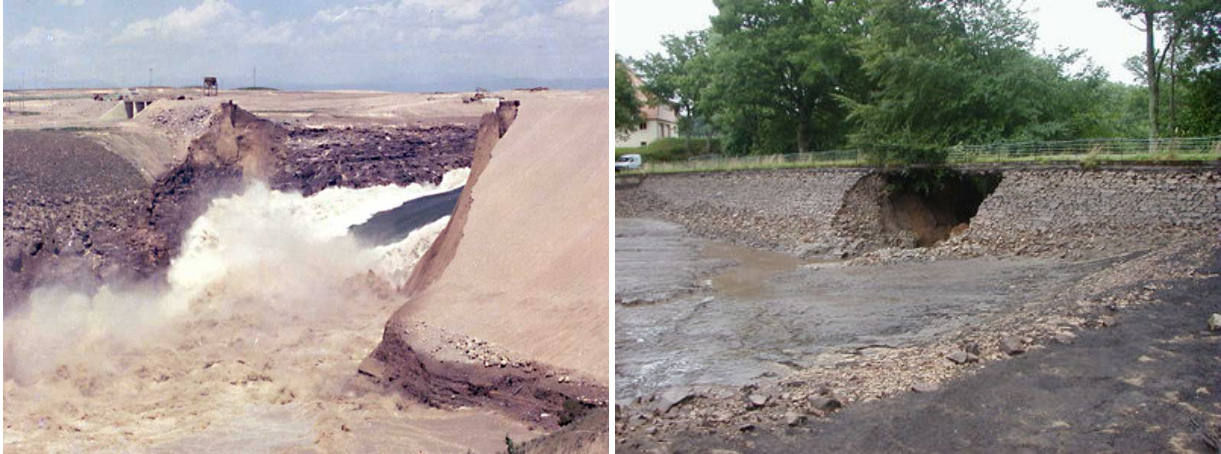
Fig. 1. (a): The catastrophic failure of the Teton dam (U.S., 1976); (b): The breach of the Ouches dam (France, 2001)
