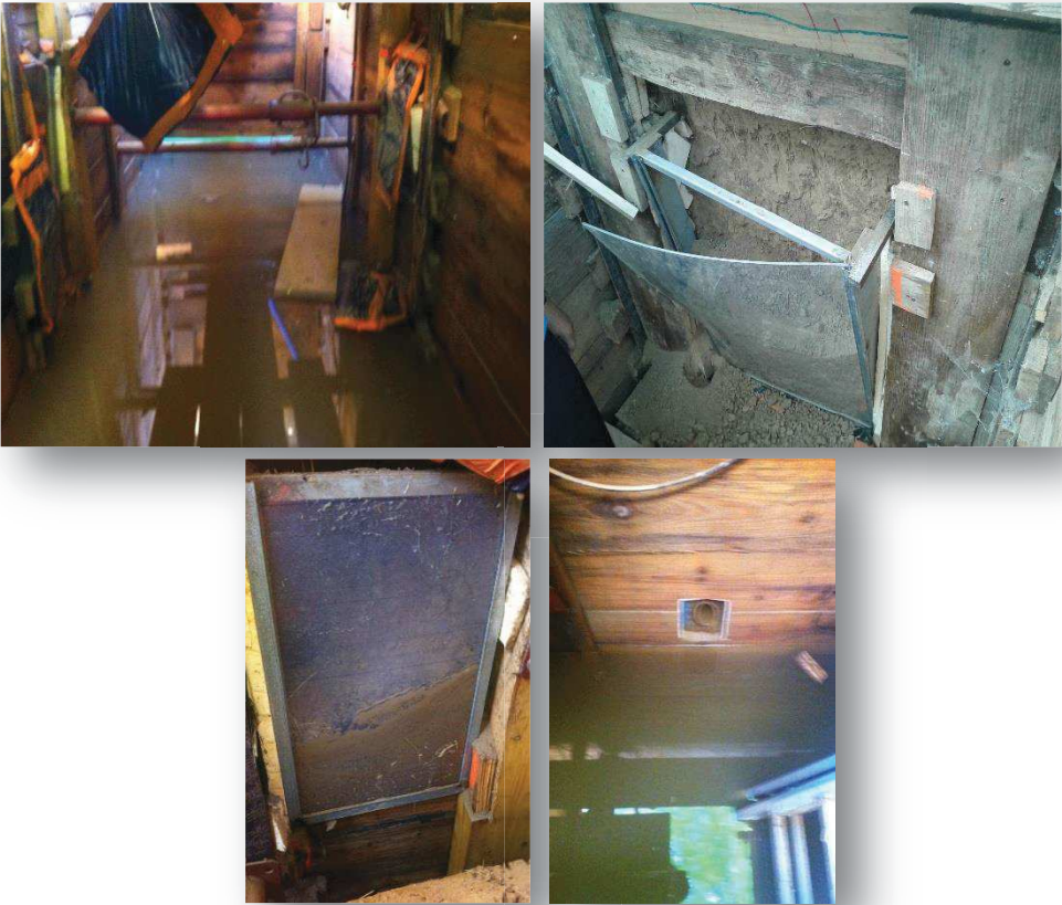
Appendix. 4: Flood damages
