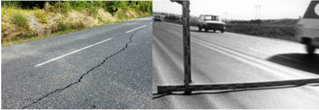
Figure 1.10 - Crack on the surface of the road on the left, small radius rutting on the right
