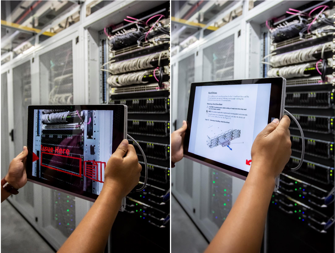
Fig. 1.1 Augmented reality for maintenance of a data center at IRT b-com.
