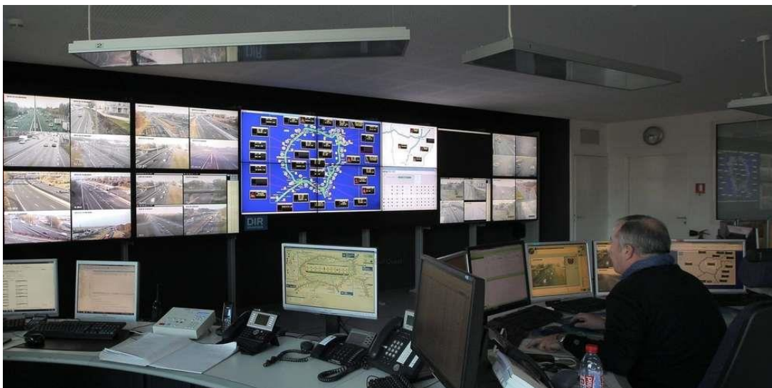
Figure 1: An operator supervising some roads in Gironde traffic management center-France 1
