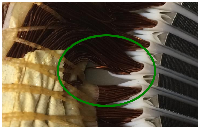
Figure 2.39. Stator winding fault in a low-voltage asynchronous motor: wire from phase V is misplaced and is in contact with a coil of phase W
