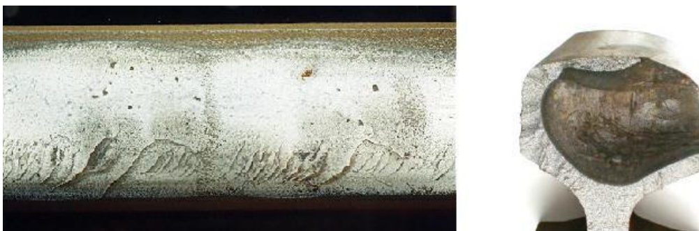
Figure 31 Severe Head Check sur rail (Dollevoet, 2010)
