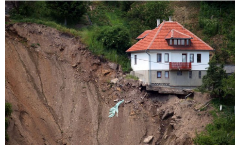
(b) Landslide in the village Željezno polje
