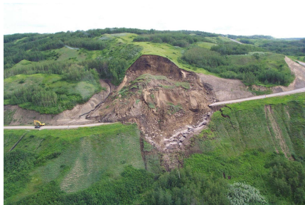
(a) Landslide on Cecil Lake Road
