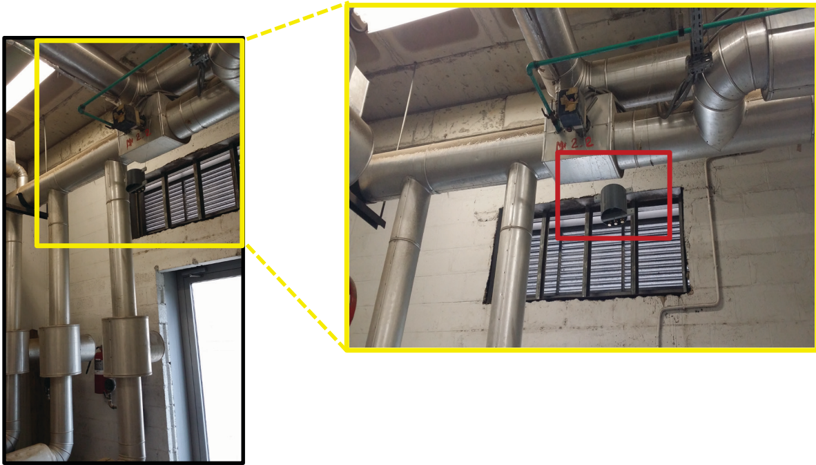
Figure 5-12: Installation of polyethylene cage (red square) in the mechanical room to measure \text{NO}_2 levels in fresh air supplying the maintenance room at Beirut Airport (November 2014)
