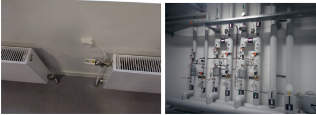
Figure 1.9 – Heating in SDU OU44 office
