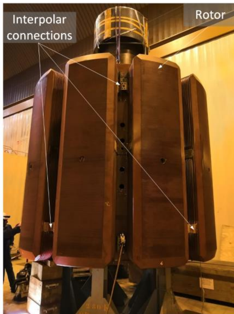
Figure 7.23: Rotor of the generator and the interpolar connections at the hydroelectric power-plant of Super-Bissorte
