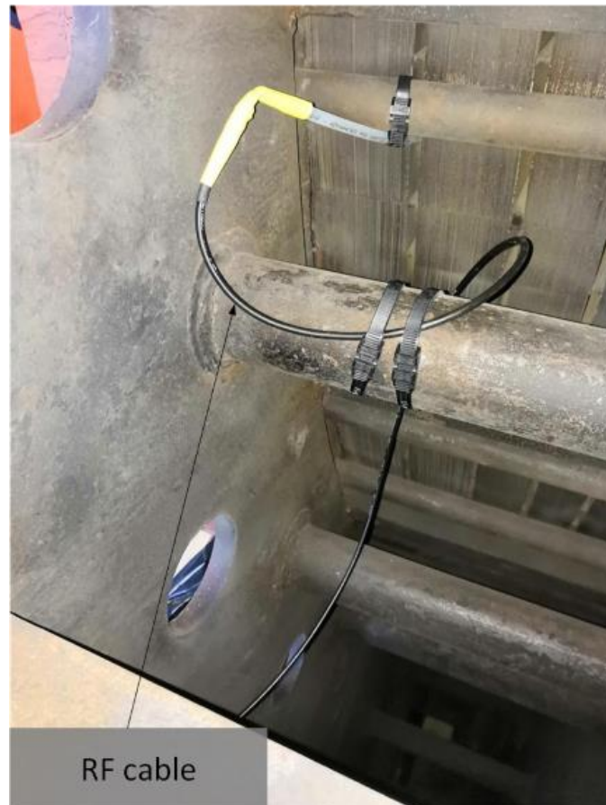
Figure 7.28: RF cable ending behind the stator
