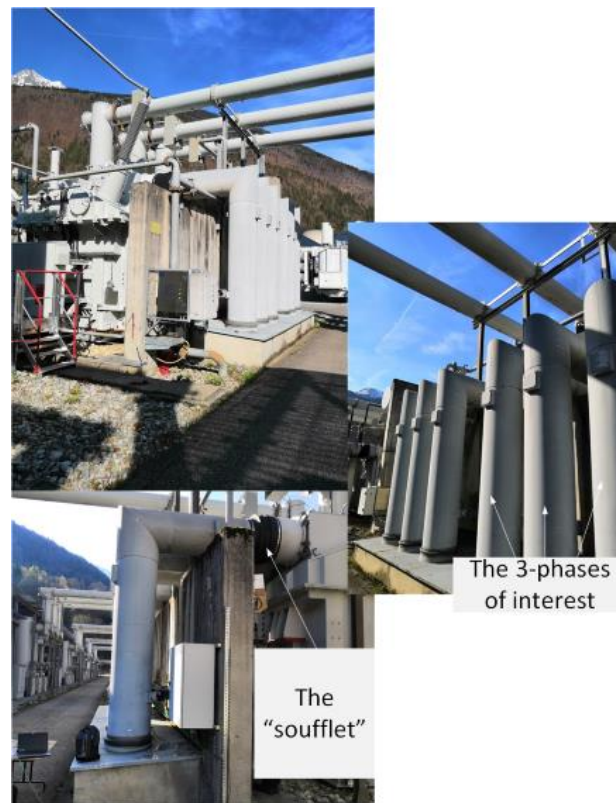
Figure 7.14: Transformers in hydroelectric power-plant of Grand'Maison
