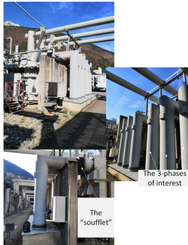
Figure 7.14: Transformers in hydroelectric power-plant of Grand'Maison
