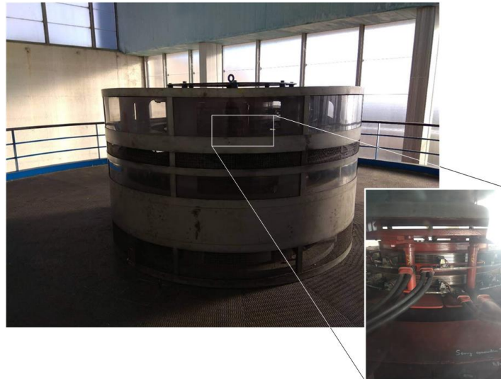
Figure 7.12: Generator at Saint-Chamas power-plant
