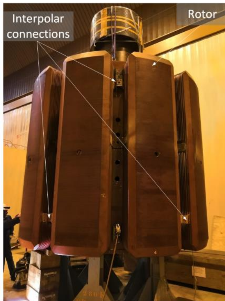
Figure 7.23: Rotor of the generator and the interpolar connections at the hydroelectric power-plant of Super-Bissorte
