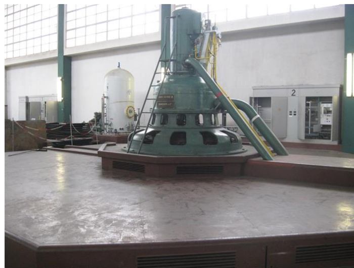
Figure 7.1: Outer view of the generator at the power-plant of Châteauneuf-sur-Isère
