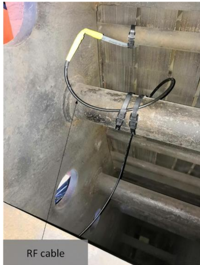
Figure 7.28: RF cable ending behind the stator
