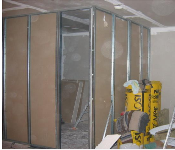
Figure 4.7. Irregular structure of the plasterboard wall
