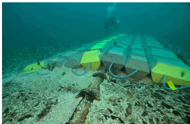
Figure 2: Photograph of iron shells and concrete mattresses used to protect an unburied cable at the tidal Paimpol-Bréhat turbine test site, France (courtesy: Olivier Dugornay, 2013).
