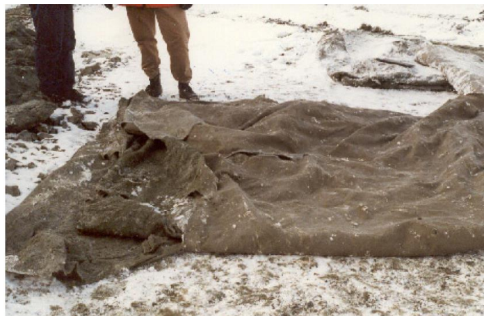
Figure 1.9-6: Geotextile damage by tear failure.
