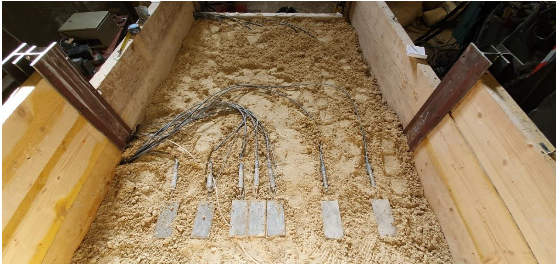
Figure 2.6-5: Illustration of the sensors installation in the traffic load test.
