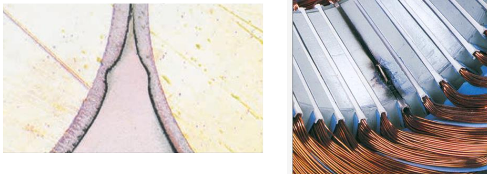
Figure 53: Consequences of PD on a stator winding insulation; left) Corroded enamel layer [40]; right) Slot liner flashover [74]
