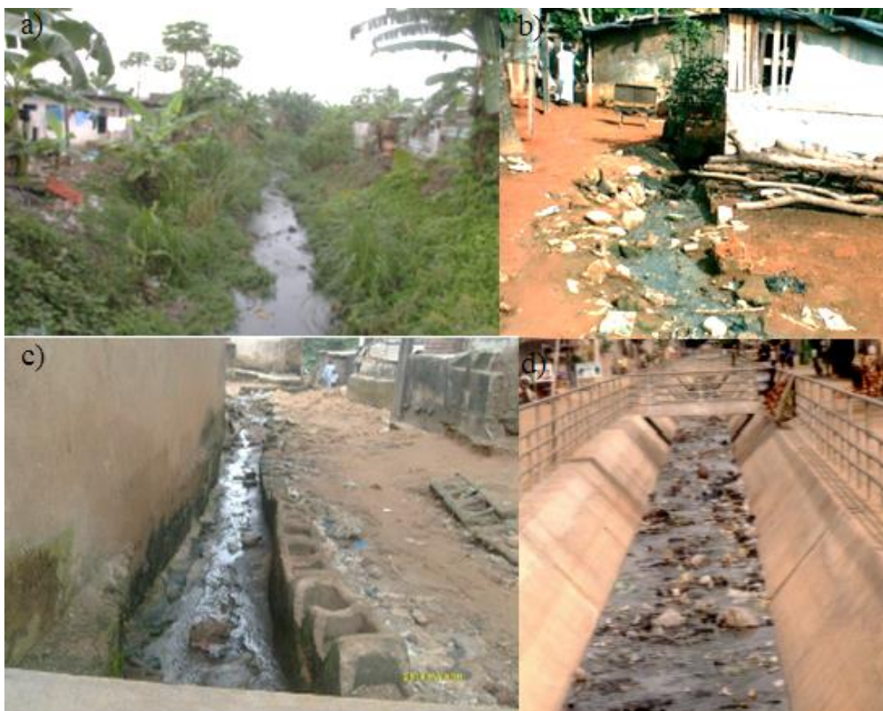
Figure 44: Inadequate sanitation systems in some cities of the West African coast. “a)” correspond to Douala (photo: Ketchemen-Tandia 2011) “b)” and “c)” correspond to Abidjan (photos credit: M. Marteau 2019) and “d)” to Cotonou (photo: Ecoloodi 2015).
