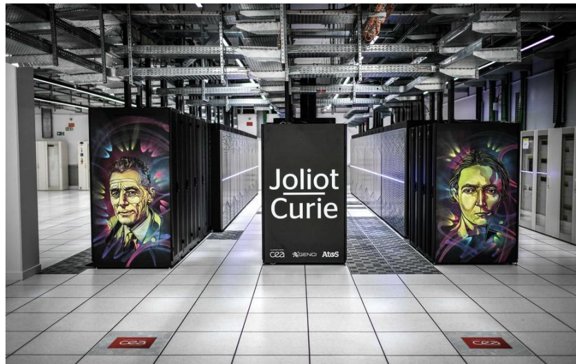
Figure 4.1: Example of a supercomputer, here Joliot-Curie at TGCC, Bruyères-le-Châtel, France
