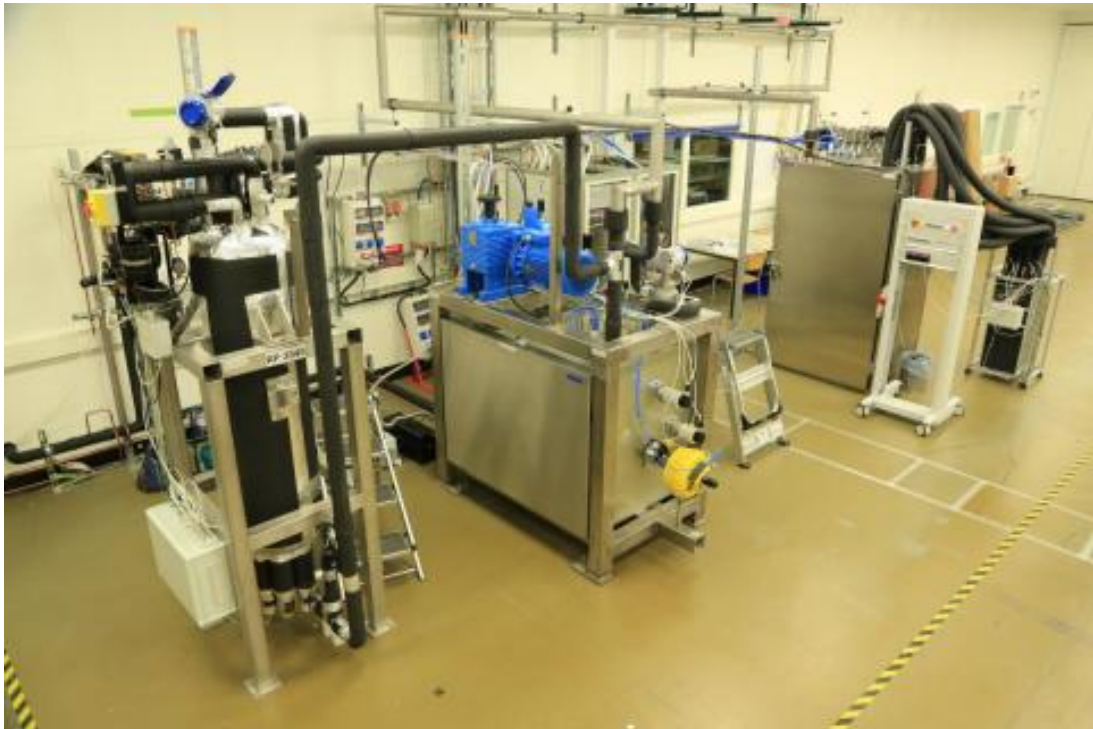
Figure 2.9: 15kW TIF plant at CERN
