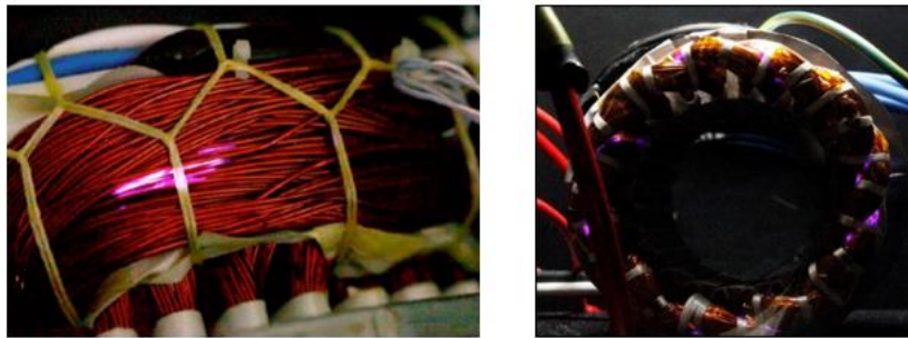
Figure I-6: Manifestation of glow PDs in end-winding and probably between phases (left) and in the stator slot (right) [9]
