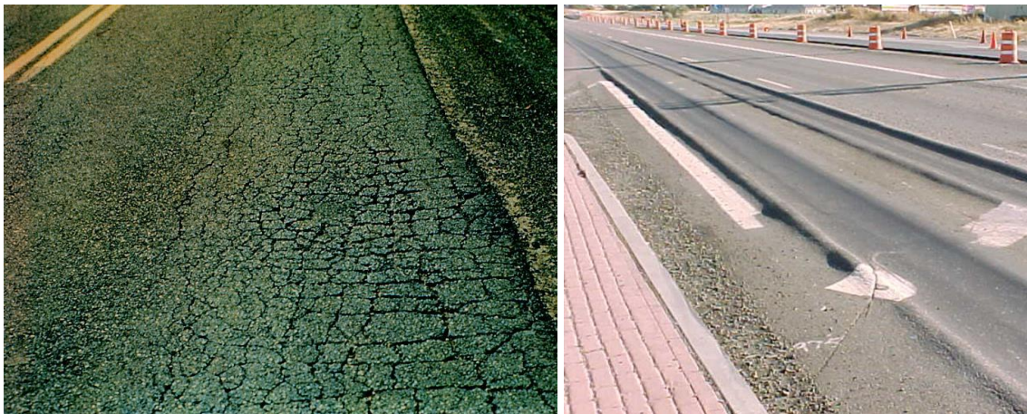
Figure 1.5 (Right) Fatigue cracking; (Left) Rutting (Source: https://pavementinteractive.org/ ).
