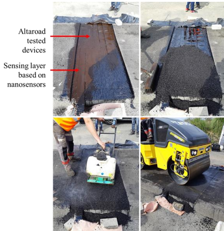
Figure 4.9 Different phases of the construction process: tack-coat emulsion application (top left), paving (top right), 1st compaction (bottom left), and 2nd compaction (bottom right).
