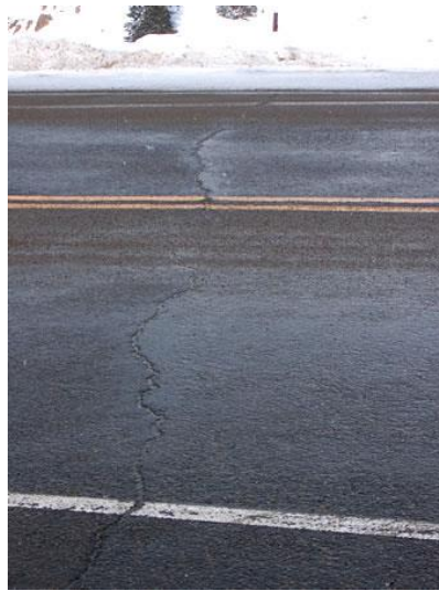
Figure 1.6 Transverse (thermal) cracking (Source: https://pavementinteractive.org/ ).
