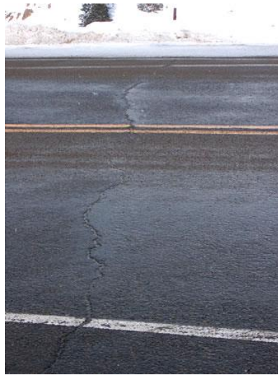
Figure 1.6 Transverse (thermal) cracking (Source: https://pavementinteractive.org/ ).
