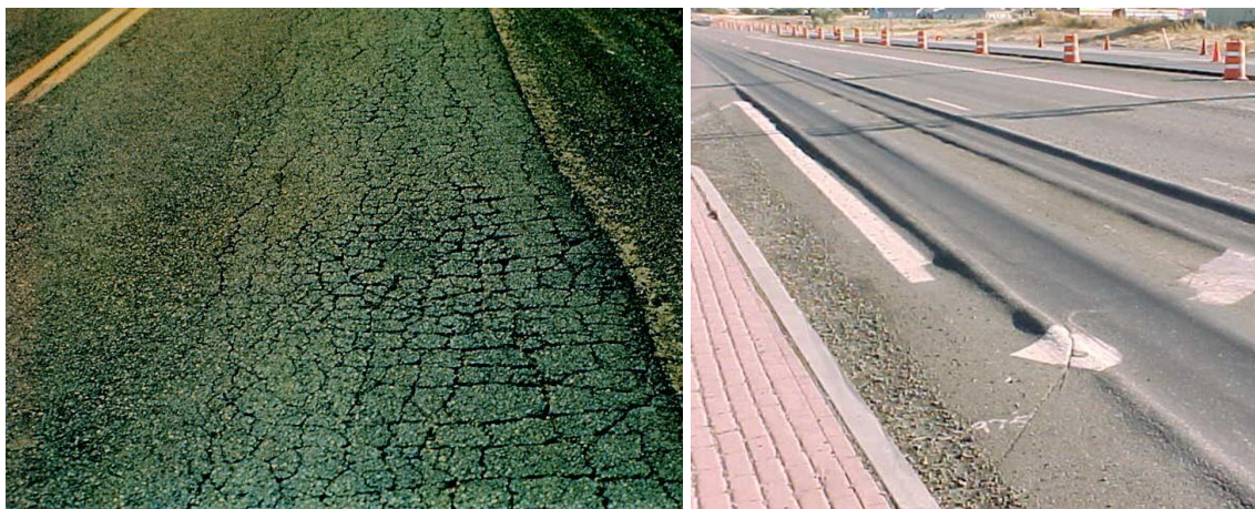
Figure 1.5 (Right) Fatigue cracking; (Left) Rutting (Source: https://pavementinteractive.org/ ).
