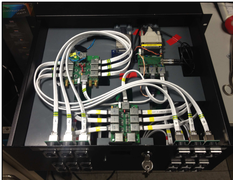
Figure 2.10: Photo of the pre-cabled 19-inch rack drawer for MIMOSA-28 setup. In the front of the box, RJ45 feed-through connectors are fixed.
