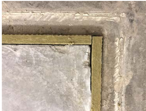
Figure 4.23: Concrete slab with mineral wool insulation placed in the gap between the perimeter of the slab and the surrounding floor at Level Acoustics & Vibration.
