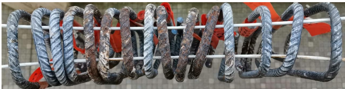
(b) Corrosion of horizontal legs in tensile zone
