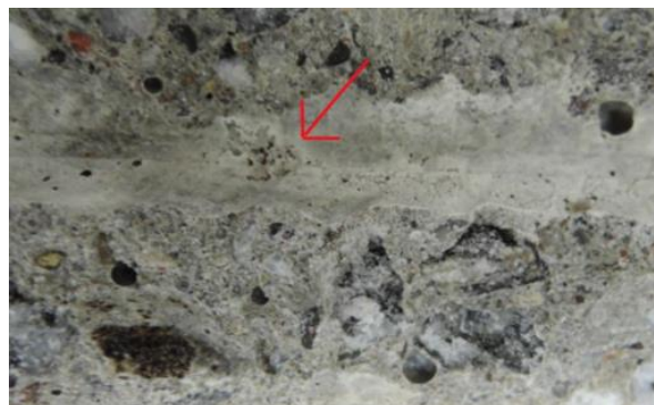
Figure II-51 Examples of irregularities at the steel-concrete interface Locally higher porosity (arrow) and small air voids (left part) as well as coarse air voids (right part). Corrosion initiated in this case at the arrow[139]
