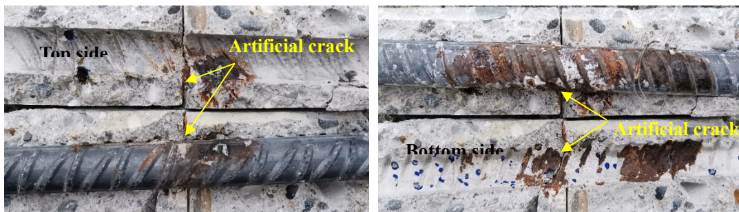
Figure IV-19. Corrosion pattern of top bar of B-1
