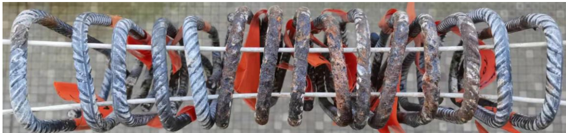
(b) Corrosion of horizontal legs in tensile zone
