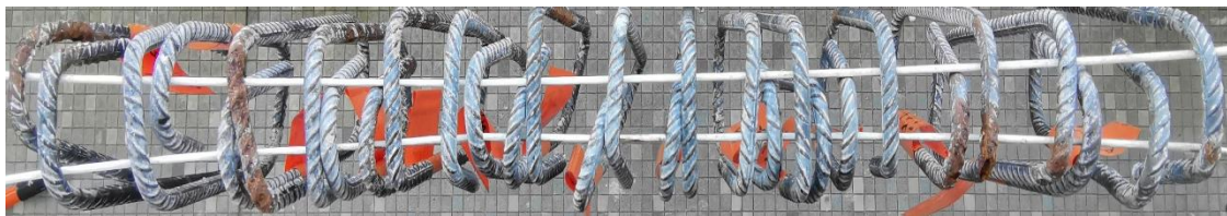
(a) Corrosion of horizontal legs in compressive zone
