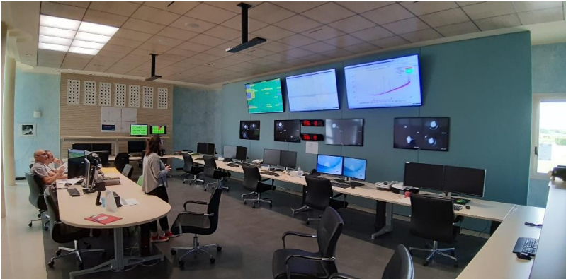
Fig. 4.6.1.b. Control Room. Source: Philippe Vincent
