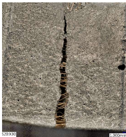
Fig. 4.22. Fibres bridging at the cracked surface of the specimen inclusion of 2% fibre loaded in opposite casting direction.
