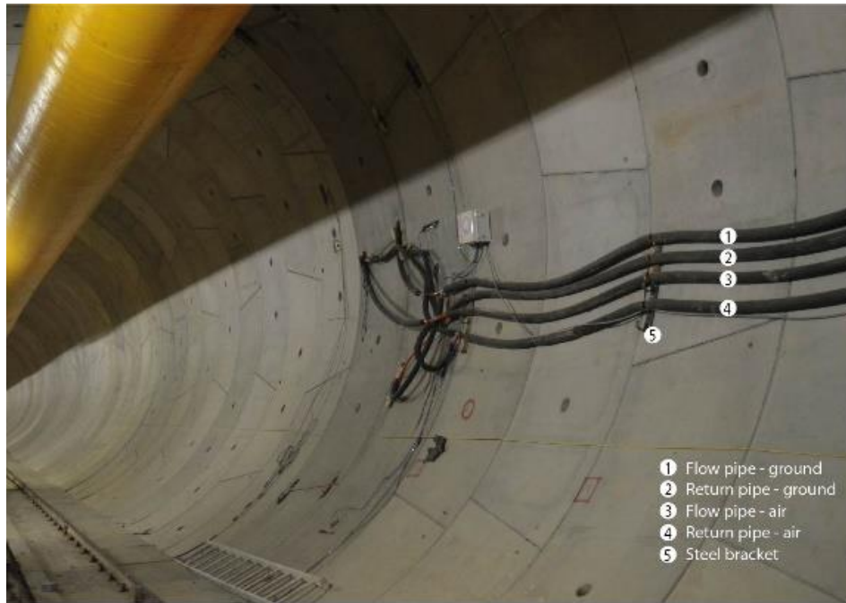
Figure 4.9: Flow and return pipes.
