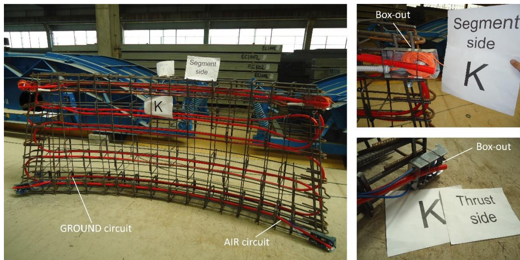
Figure 4.6: Example of steel cage equipped with pipes before casting (segment 1, ring 180) with detail of box-outs.
