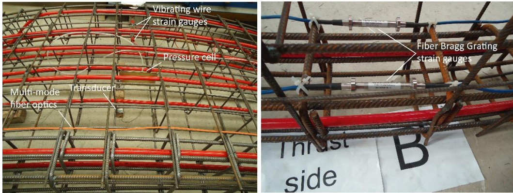
Figure 4.14: Energy segments equipped with the three types of monitoring system.
