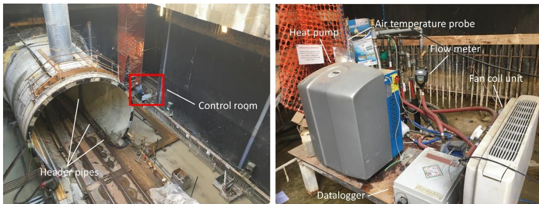
Figure 4.11: The control room, hosting the heat pump, the datalogger and the secondary circuit, view from the mezzanine (left) and a close-up view (right).
