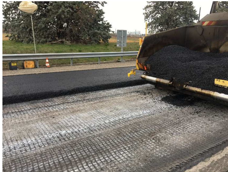
Figure 2-26. Construction site with use of fiberglass geogrid solution to reinforce the highway A7 in Montélimar in 2018 by EIFFAGE Infrastructures using the fiberglass geogrid Notex Glass C ® provided by Afitexinov
