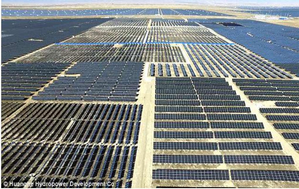
FIGURE 8: Longyangxia Dam solar park.
