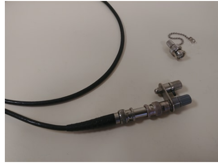
(b) Faulty termination.
