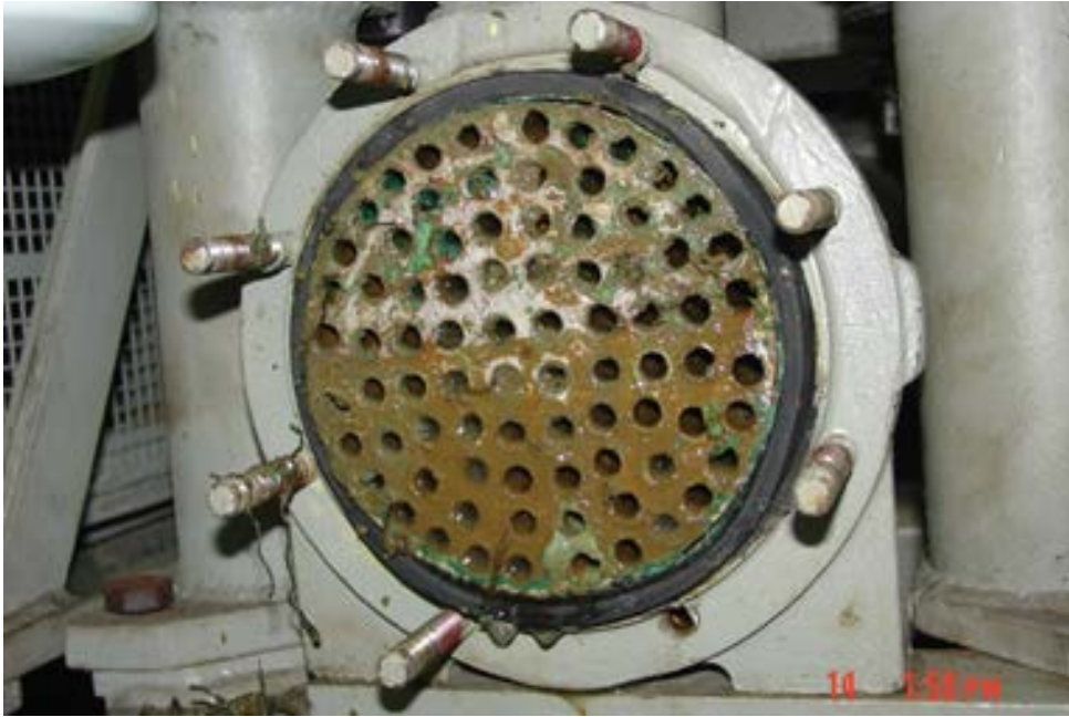
FIGURE 1.1 – Photo of fouled inner surfaces of tubular heat exchanger used in a ship (Navy Currents Winter 2015)
