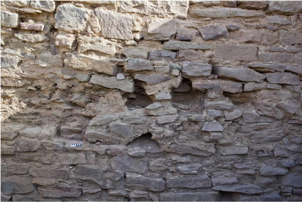
Figure 25: Wall SU 3969 with beam holes facing the entrance of Building F-b3 in the N; view from S (© DAI Orient Department 2011 F. Weigel)
