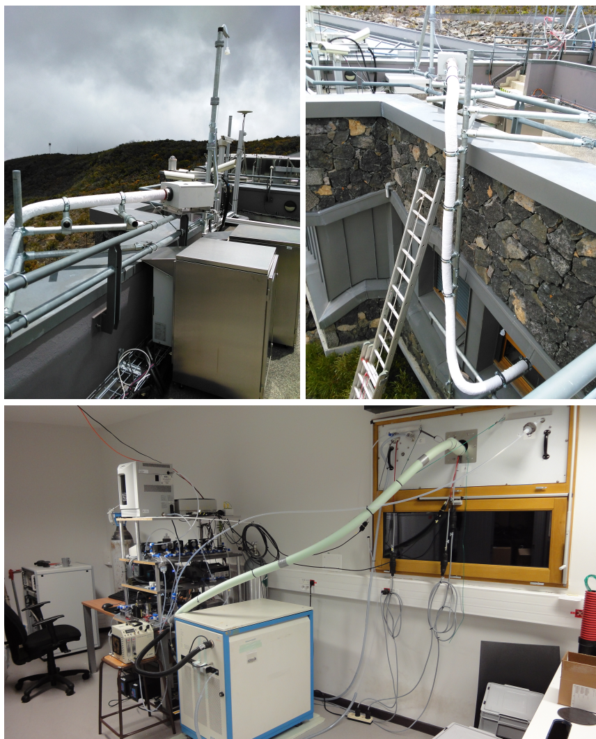
Figure 3.2: Top left: sampling point on top of the roof of the Maïdo observatory together with the filter box after which the sampling line is thermally insulated and heated by a few degrees above ambient temperatures. Top right: heated sampling line from the filter box towards the window of the observatory. Bottom: sampling line entering the laboratory through a custom board replacing the window and connecting to the manifold which controls the air flow towards the hs-PTR-Quad-MS. Photos by C. Amelynck.
