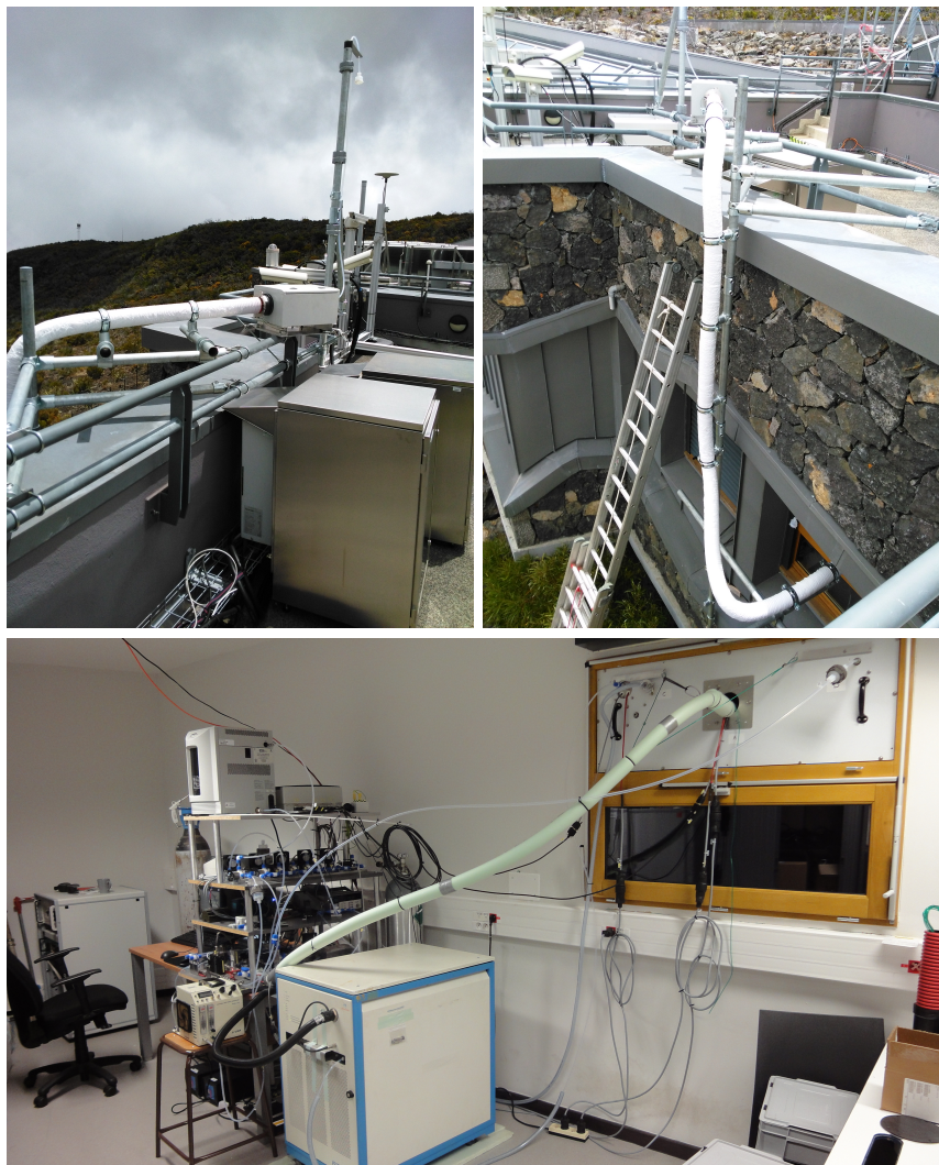
Figure 3.2: Top left: sampling point on top of the roof of the Maïdo observatory together with the filter box after which the sampling line is thermally insulated and heated by a few degrees above ambient temperatures. Top right: heated sampling line from the filter box towards the window of the observatory. Bottom: sampling line entering the laboratory through a custom board replacing the window and connecting to the manifold which controls the air flow towards the hs-PTR-Quad-MS. Photos by C. Amelynck.
