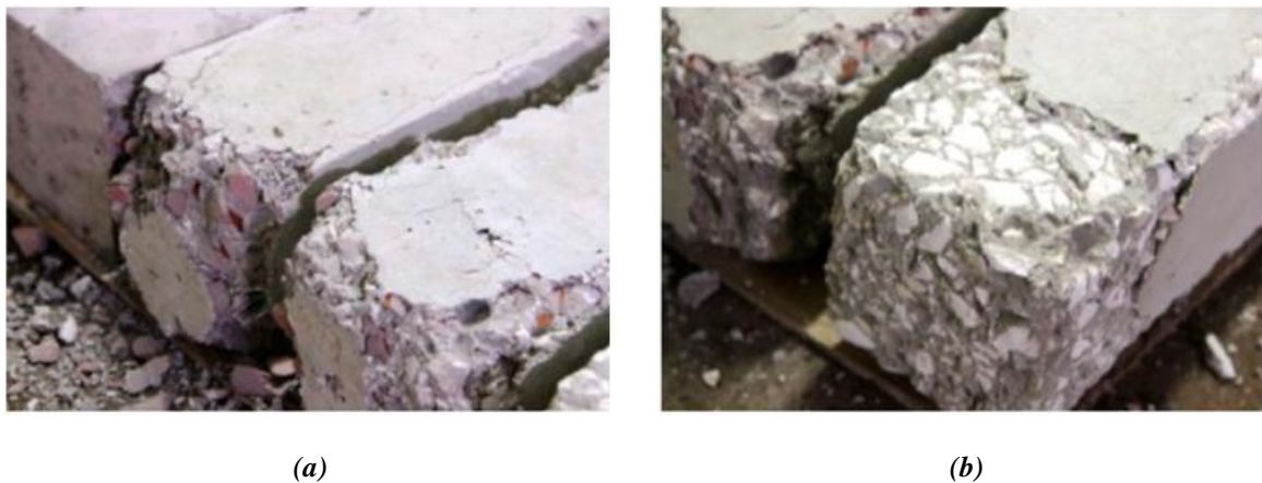
Figure I.4 The difference of surface spalling, after exposure to a temperature of 1000 °C, between (a) concrete containing crushed bricks and roof tiles aggregates and (b) concrete containing crushed basaltic aggregates ( Miličević et al., 2016 )
