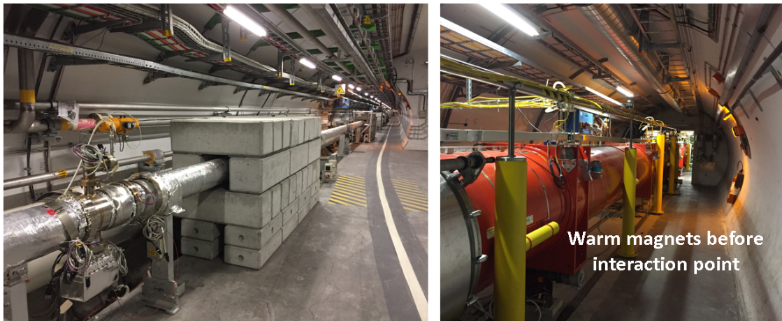
Figure 2.10: Photograph of the Long Straight Section (LSS) before the CMS experiment in 2019.
