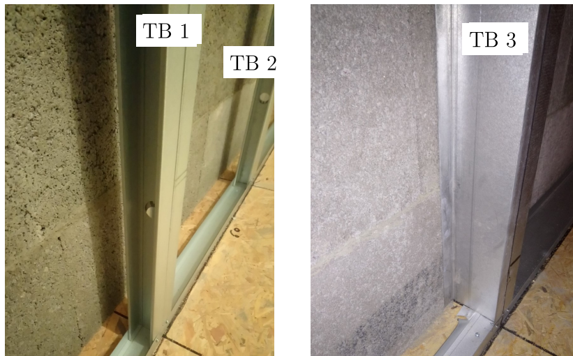
Figure 4.16.: CEREMA: Pictures of metal rails used to hold the insulation system (thermal bridges).
