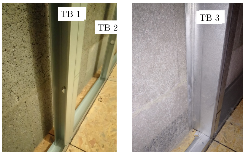
Figure 4.16.: CEREMA: Pictures of metal rails used to hold the insulation system (thermal bridges).
