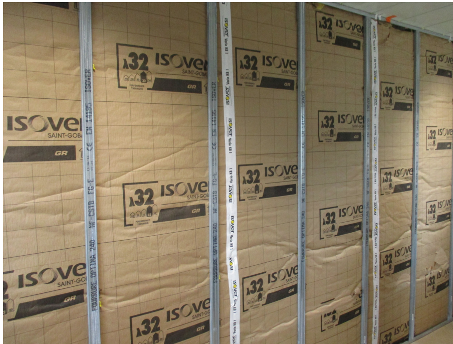
Figure 4.26.: SGR: Picture of the North wall insulation system.
