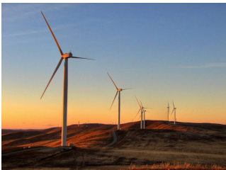
(c) Wind turbines
