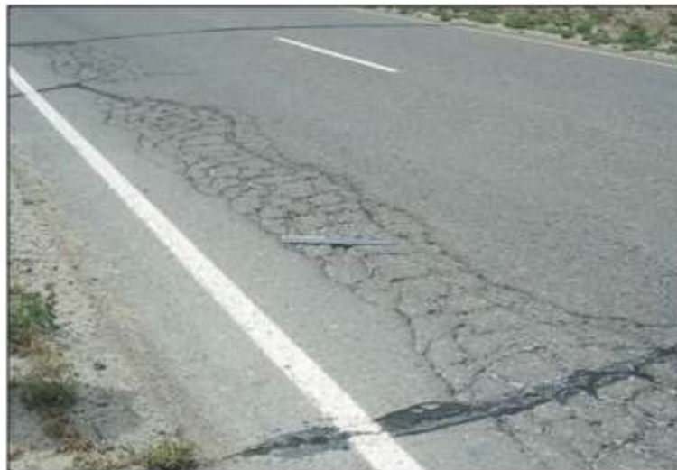
Figure 2-9 Example of severe fatigue cracking (Miller and Bellinger 2014)
